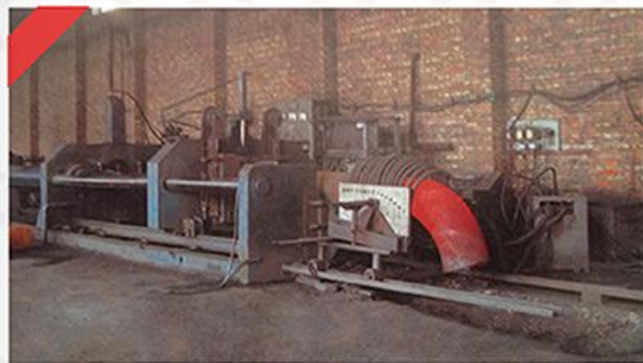
推制一, 三车间 NO. 1 AND 3 EXTRUDING WORKSHOP
